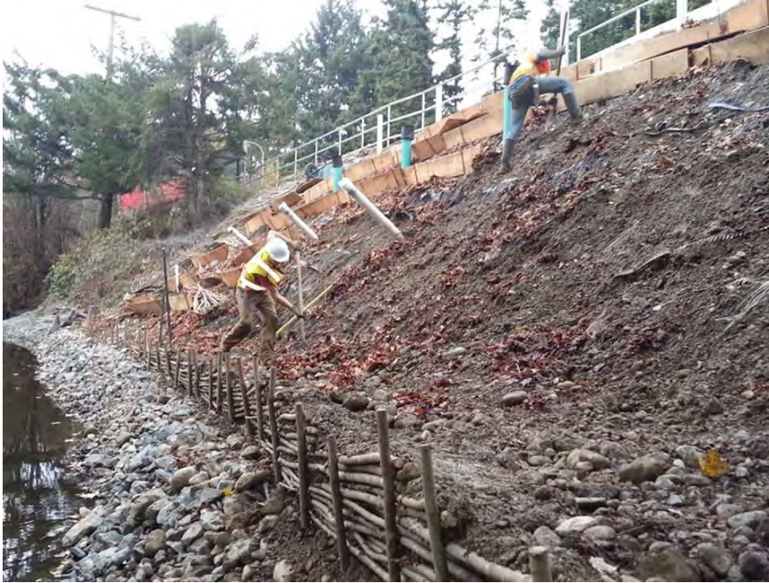
Photo 4. Willow crib wall being installed to replace the failed treatment show in Photo 2.
