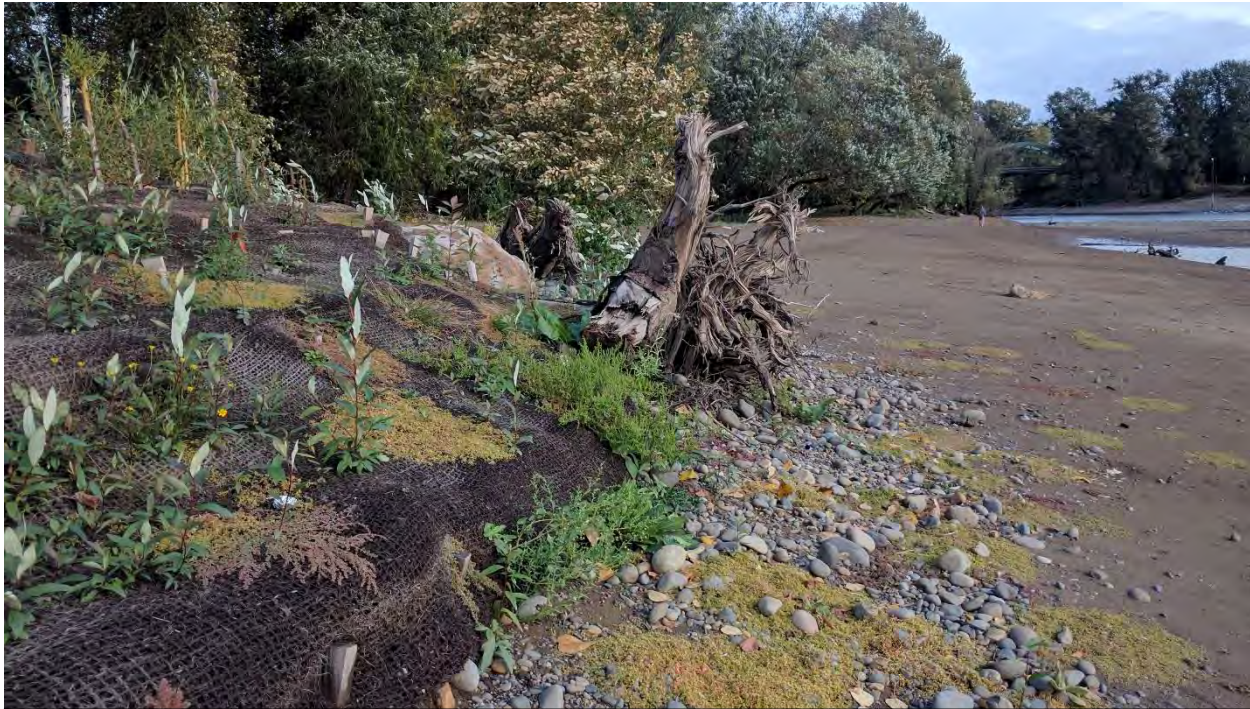
Photo 3. Dahl Beach Mitigation South Site, one year after installation. The upstream rootwads and anchor rocks can be seen. Willow and other plants are beginning to establish through the coir woven mesh blanket. ETC Photo 10/20/2017.
