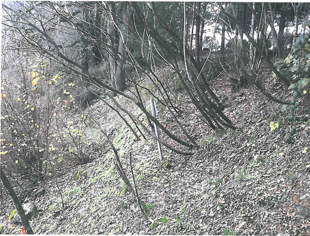
Photograph 3 - Looking southwest on slope. Note the scarp and slumping area in the location of the signpost.
