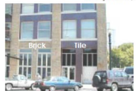
Not Recommended: Facade of historic building is marred by addition of a brightly colored contemporary tile cladding (SW Salmon and 11th, Portland)
