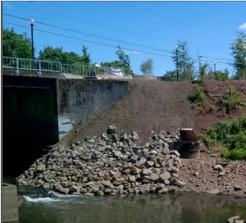
Figure 5. Existing bridge with slope scour
