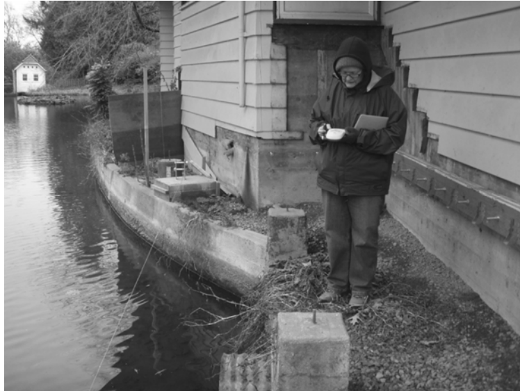
Figure 7. View to north of area behind Pond House in which replacement deck will be installed. Plans (Figure 1A) call for stairs to extend from doorway behind person down to deck (see prior stair and deck supports on back wall of house) with a second set of stairs extending away from the camera along the back wall to the north. Note Spring House in background (white building). This is where the section of Spring Creek that is piped under Harrison is discharged. Flow is to north away from viewer.
